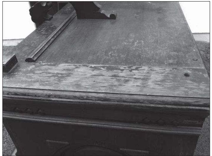
Finish as found, in bad condition.
